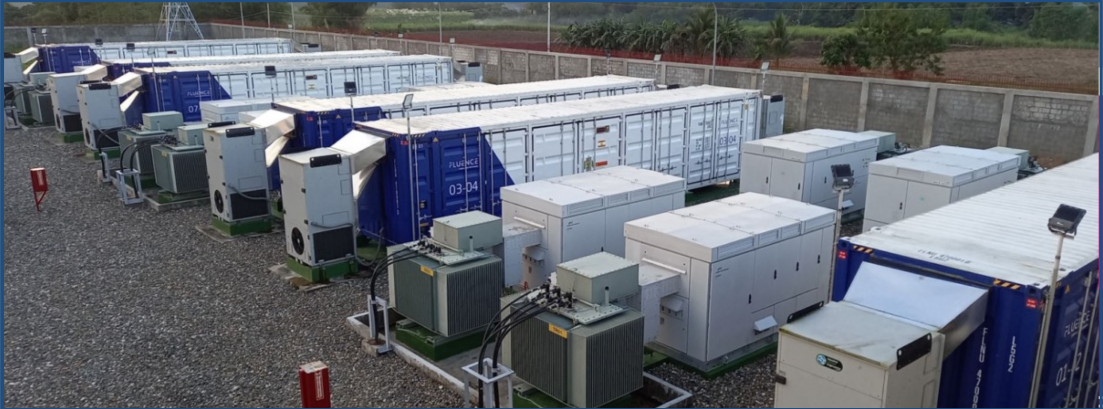
Battery Energy Storage System
